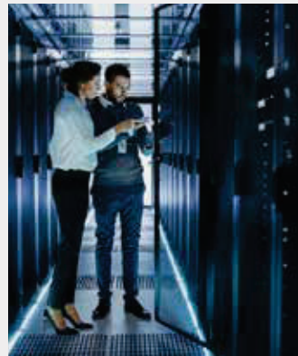
Instant data center
